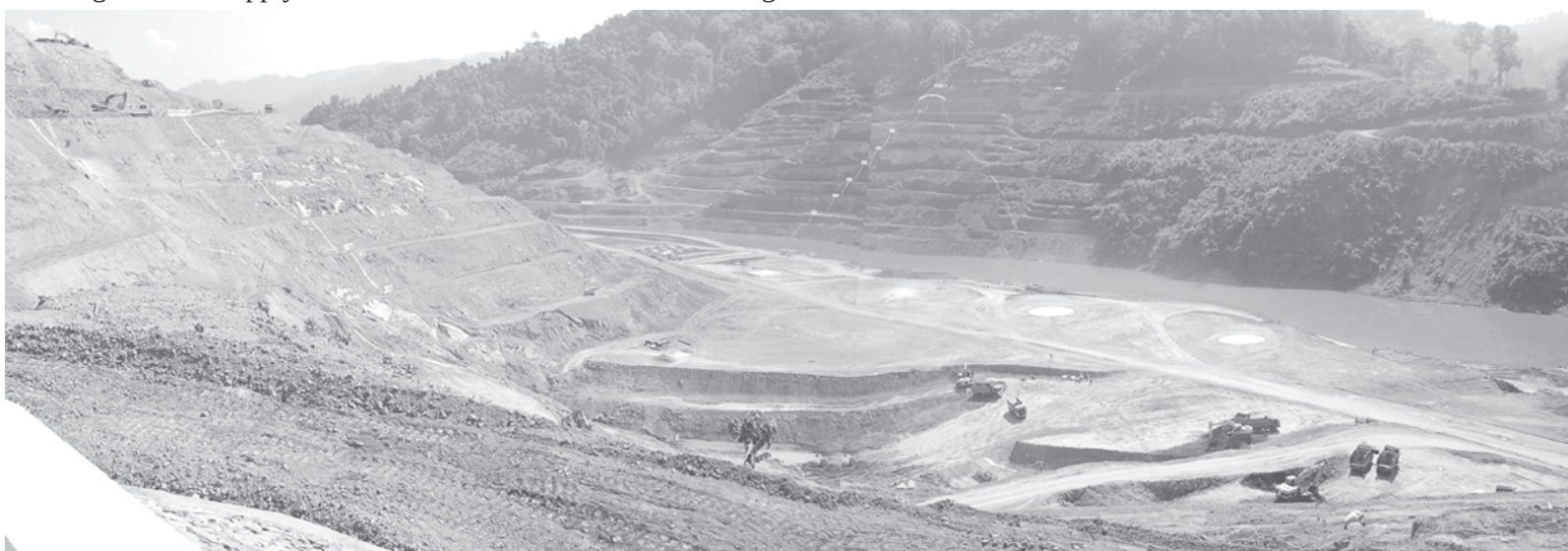
Thahtay Creek hydropower project in Rakhine State.—MNA
