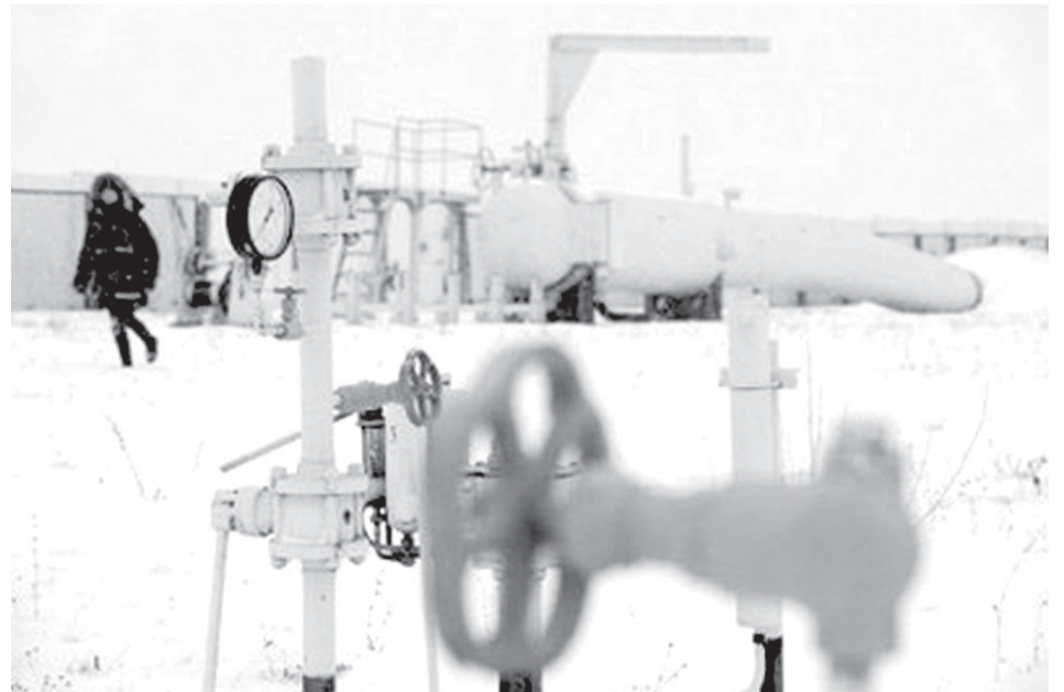
A woman passes by a gas pipe of the gas-compressor station in the small Ukrainian city of Boyarka, near Kiev on 4 January. Ukraine said on Tuesday that Russia had drastically cut gas supplies to Europe and warned of "problems" ahead as several European countries reported that deliveries of Russian gas had stopped.—INTERNET
