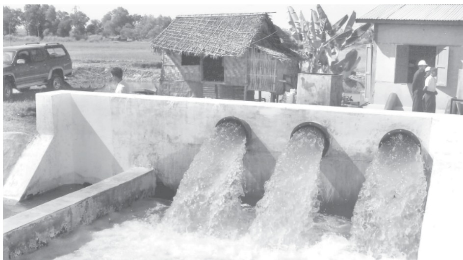
Water is pumped to main canal with the use of paddy husk-fired power at Balar Water Pumping Station.
