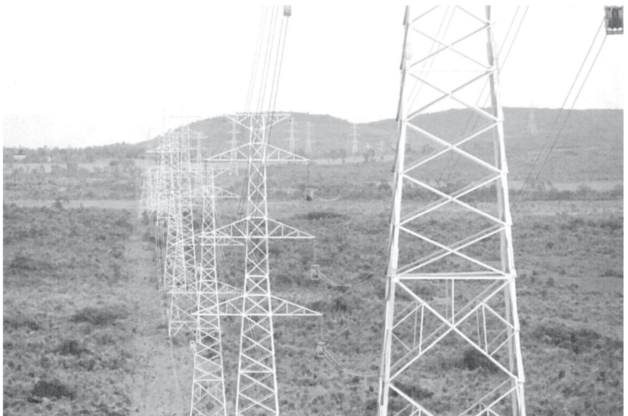
Nawnghkio detour power line of Mansan-Shwesaryan section.
