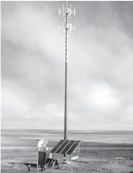
Workers man a China Mobile relay station near the Qinghai-Tibet railway.—INTERNET
