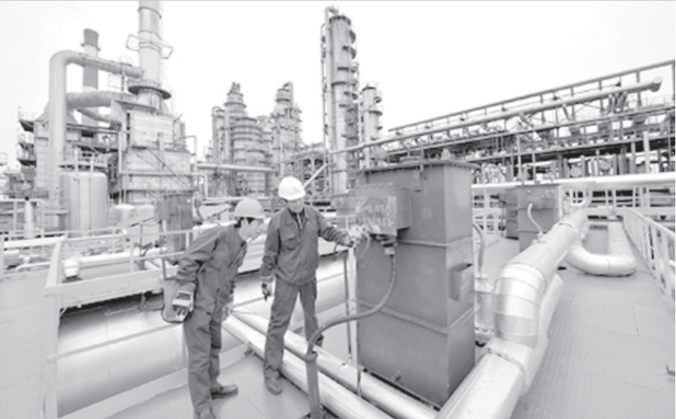
Two technicians check the equipments in an oil refinery of China Petroleum and Chemical Corporation (Sinopec) in Ningbo, east China’s Zhejiang Province, on 29 March, 2008.—XINHUA
