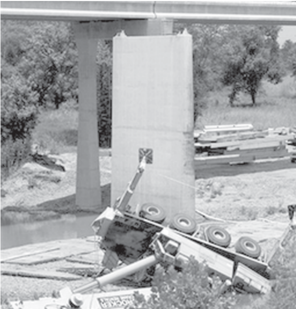
A toppled mobile crane, the base for which rests almost upside down on a man-made support in the Colorado River is shown after the accident on 30 July, 2008, in Smithville, Texas. Workers were attempting to remove parts of the old bridge, the support for which is shown in the center. —INTERNET
