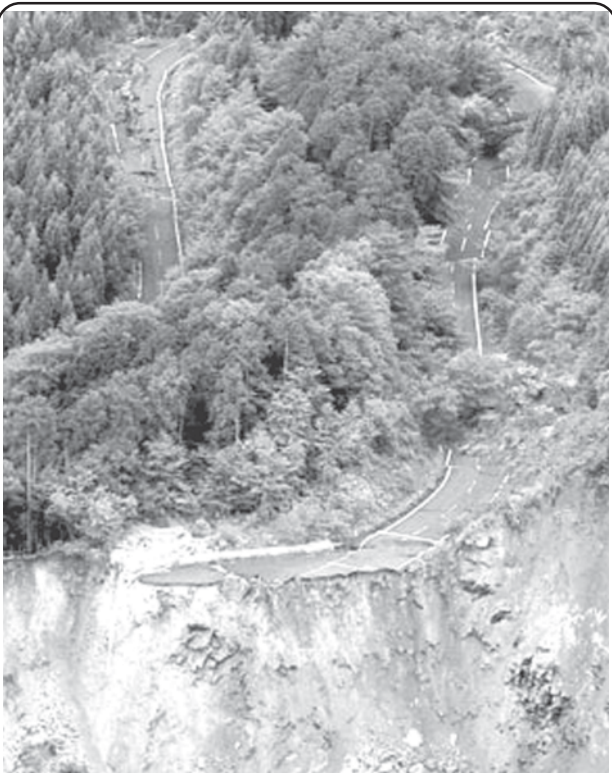
A road destroyed by an earthquake is pictured near Kurihara City, Miyagi Prefecture on 14 June, 2008.—XINHUA
