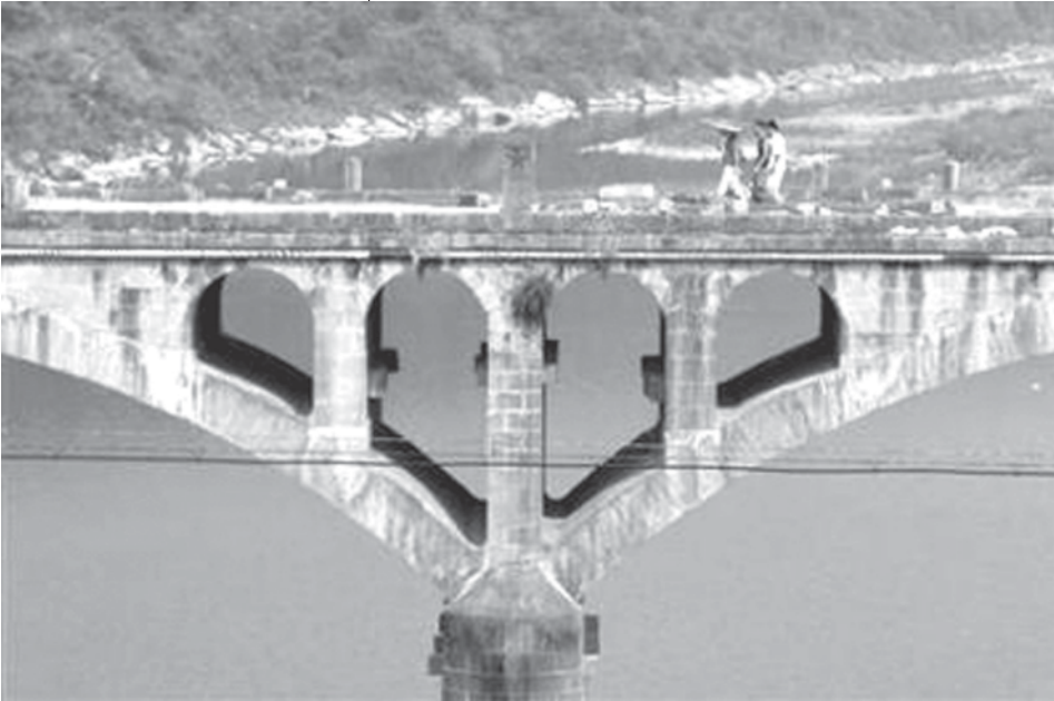
Residents walk across a damaged bridge over the Pen Jiang River which connects to the Tangjiashan quake-lake in Qinglian town of earthquake-hit Jiangyou county, Sichuan Province on 5 June, 2008.—INTERNET
