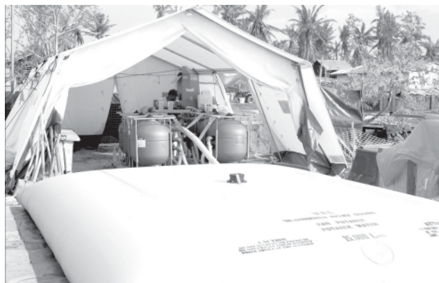
A water purifier installed in the relief camp in Yadana Dipa sports grounds.
