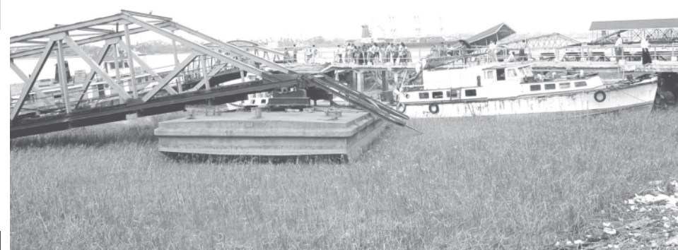
Damaged wharf at Botahtaung jetty.—MNA
