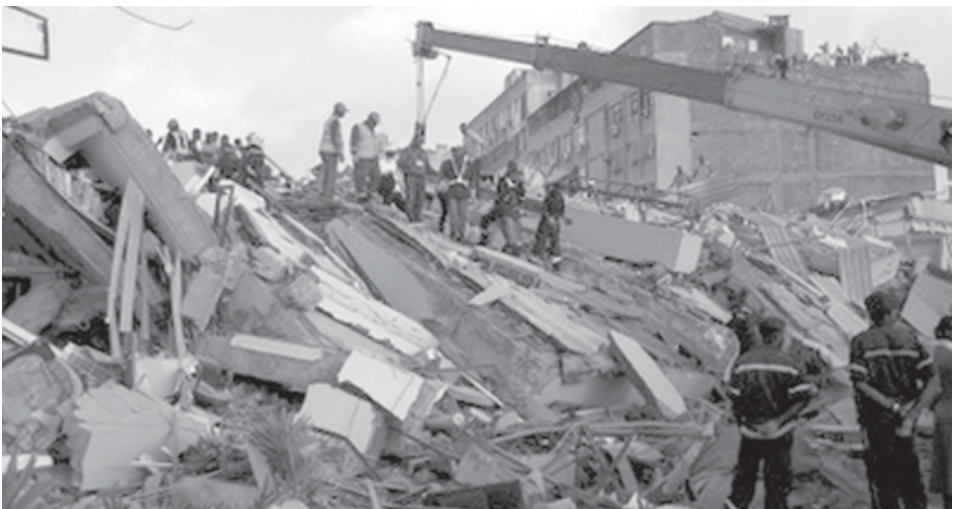
Angolan rescue workers and policemen work on the site of the collapsed criminal investigation department building in Luanda on 29 March, 2008. —XINHUA
