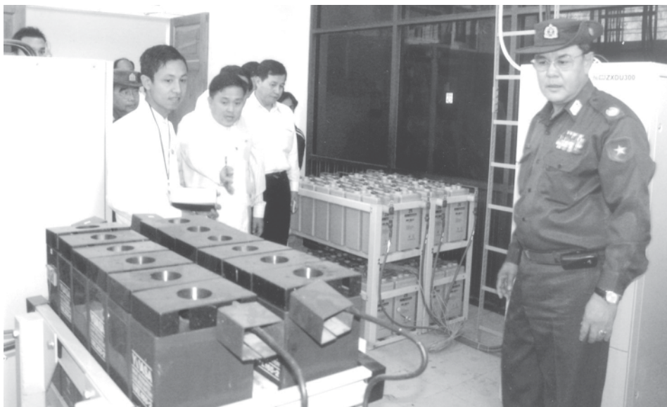
Minister Brig-Gen Thein Zaw inspects communication station in Myitkyina. — CPT
