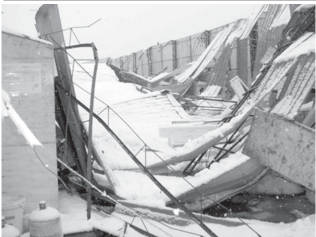
Remains of a factory outside Shanghai, devastated by violent snow storms which have hit China on 31 Jan, 2008.—INTERNET
