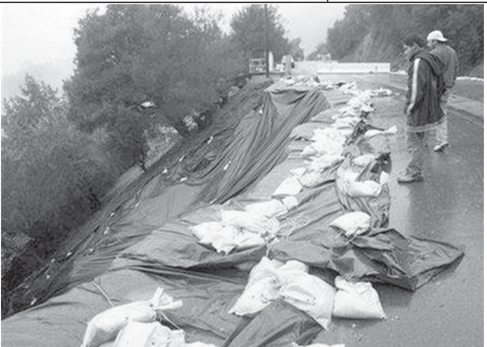
People look at a road damaged as a result of a mudslide in Oakland, California on 5 Jan, 2008. Storms battered the western United States on Saturday with strong winds, heavy rains and a blanket of snow that caused widespread power outages, a levee break in Nevada and two deaths in California.—INTERNET
