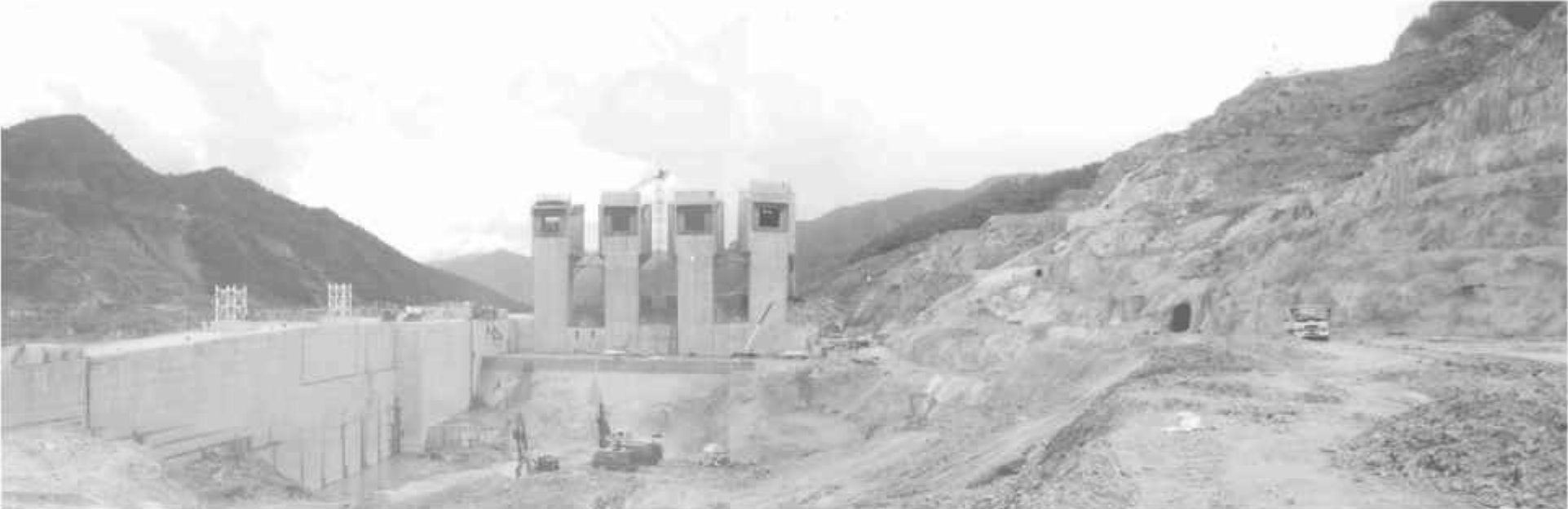
Yeywa Hydrel Power Project. — ELECTRIC POWER-1
