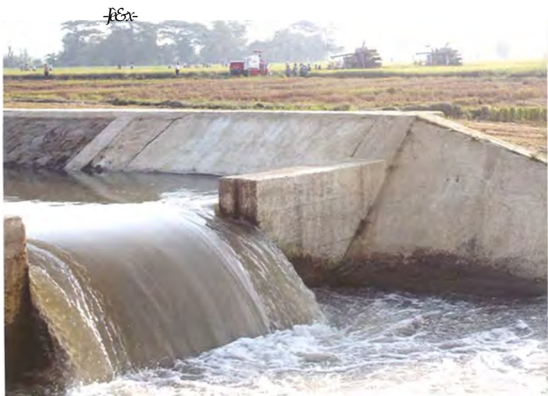
Constructed River Water Pumping Projects
