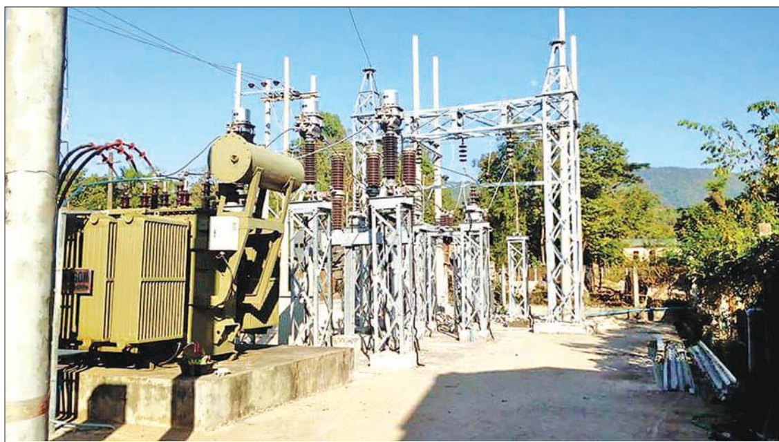
Kyaukkyi Electric Transformer. PHOTO 045 (KYEMON)
