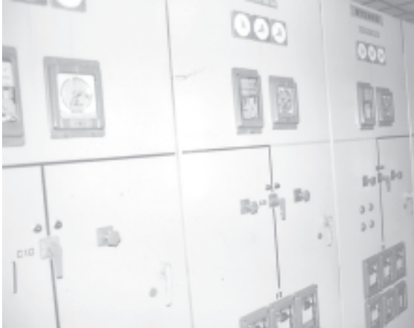
Lt-Gen Kyaw Win inspects sub-power station of the Ministry of Electric Power in Pathein, Ayeyawaddy Division. —MNA
