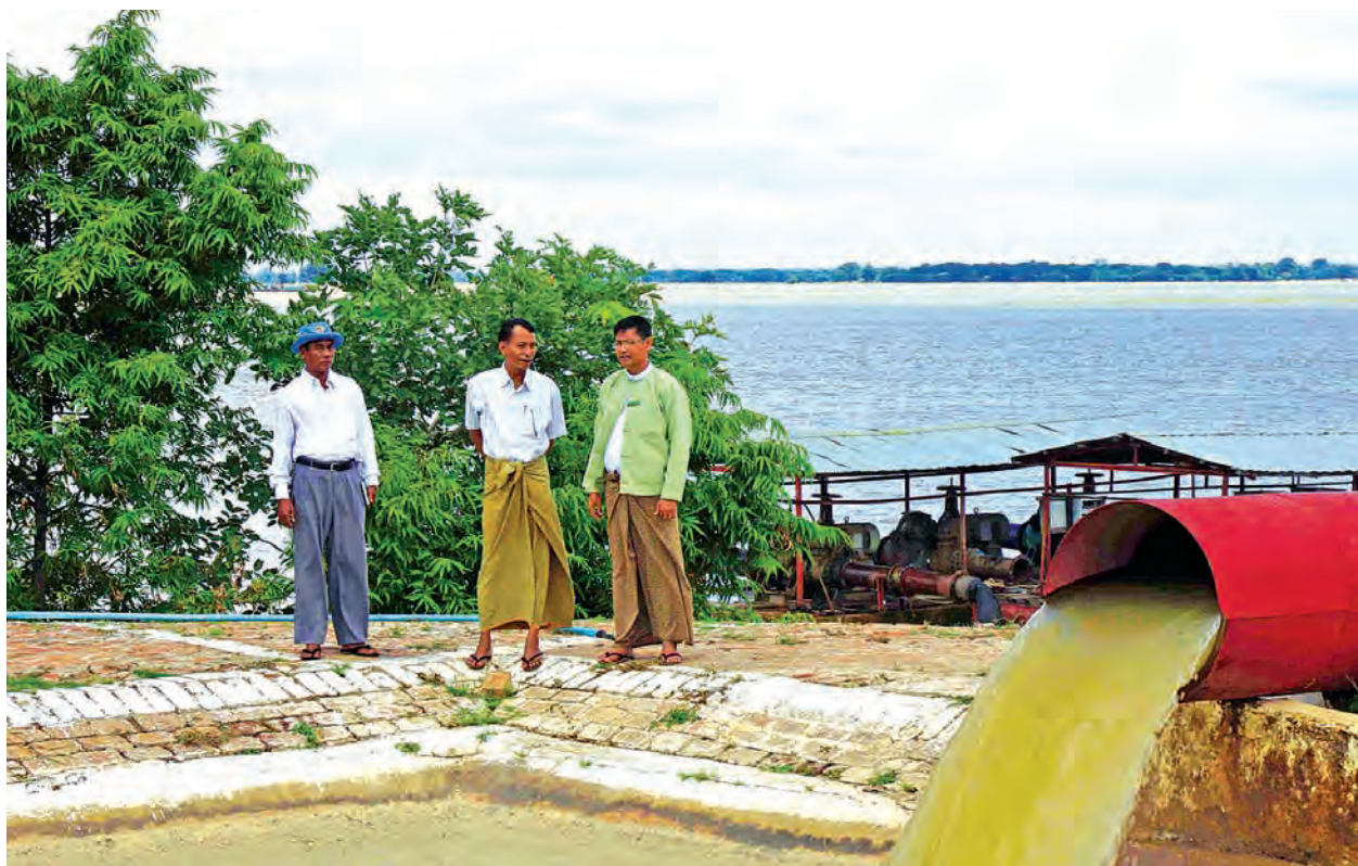
River water pumping station pumping water from Ayeyawady River to feeder canal.
