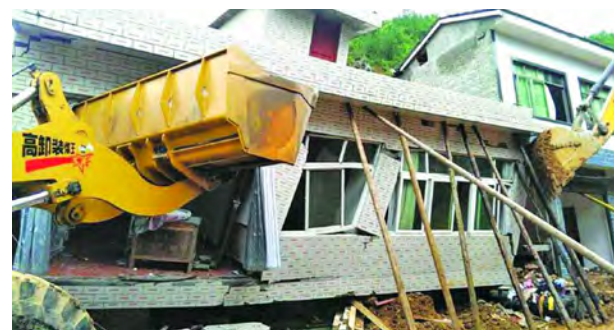
Two residential buildings are damaged by landslide in Dakuo Village of Zhijin County in Bijie City, southwest China's Guizhou Province, on 17 July, 2014. — XINHUA
