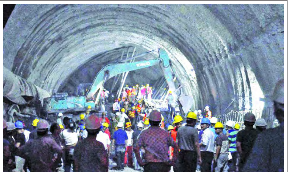
Rescuers work in a collapsed railway tunnel in Funing, southwest China's Yunnan Province, 15 July, 2014. Rescuers were working all out Monday night hoping to reach the 15 workers who had been trapped in the debris of the collapsed railway tunnel in Funing County. The tunnel, known as Funing No 1 tunnel, was on a 710-km railway linking Kunming with Nanning, capital of the neighbouring Guangxi Zhuang Autonomous Region. Part of the tunnel, which was still under construction, collapsed at 4 pm on Monday.—XINHUA
