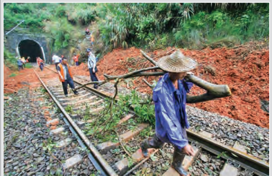
Rescuers clean tree branches from the railway in southeast China's Fujian Province, on 20 June, 2014. A total of three sections of the railway linking Shaowu and Shunchang in Fujian Province were blocked by landslides, two of which have been resumed to service.—XINHUA
