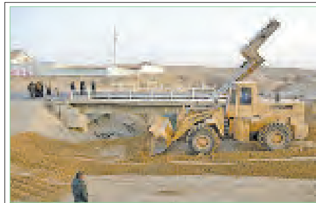
A bulldozer works to open an alternative pathway beside the crushed bridge on the No. 304 Provincial Highway, the Shuitao Village, Hongsibao District of Wuzhong City, northwest China's Ningxia Hui Autonomous Region, on 10 Feb, 2013. According to local highway authorities, an overloaded truck carrying the outsized casting, with a gross weight of 100 tons, crushed the bridge with design load of only 55 tons when the truck tried to pass over it. —XINHUA
