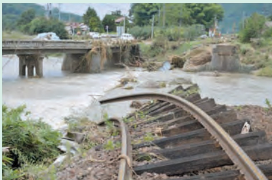
Photo taken on 29 July, 2013, shows railway track on the JR Yamaguchi Line severed by a swollen river after heavy rain in Yamaguchi City in Yamaguchi Prefecture, western Japan. — KYODO NEWS
