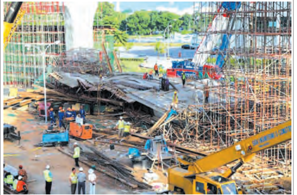
Workers of a rescue team work at the site of the collapsed bridge in the northeastern state of Penang, Malaysia, on 7 June, 2013. An interchange ramp to a cross-sea bridge that is under construction in northern Malaysia collapsed on Thursday, and rescue teams are still searching for survivors who might be trapped under the debris.—XINHUA
