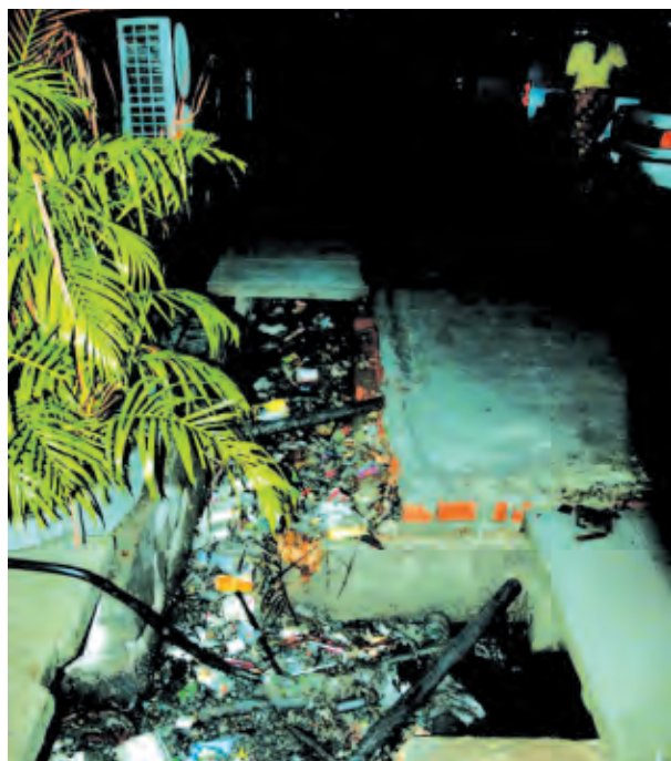
Photo shows an underground drain choked with rubbish at the corner of Botahtaung Pagoda Road and Maha Bandoola Street.
