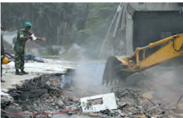
Rescue workers attempt to find survivors from the rubble of the collapsed Rana Plaza building in Savar, around 30 km (19 miles) outside Dhaka on 4 May, 2013.
