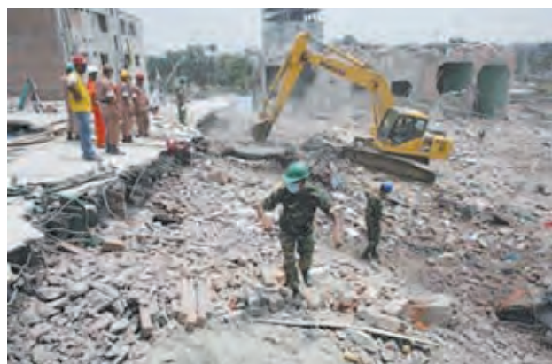
Rescue workers attempt to find survivors from the rubble of the collapsed Rana Plaza building in Savar, around 30 km (19 miles) outside Dhaka on 4 May, 2013. — REUTERS
