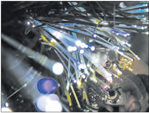
Fiber Optic Cables
