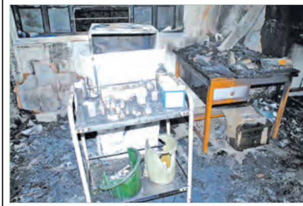
Fire damage is seen at the nursery ward of PBM Government Hospital in Bikaner, India, on 13 Jan, 2013. A fire broke out on early Sunday morning due to a short circuit in the air-conditioner at the nursery ward of PBM Government Hospital in Bikaner where three children were injured.— Xinhua
