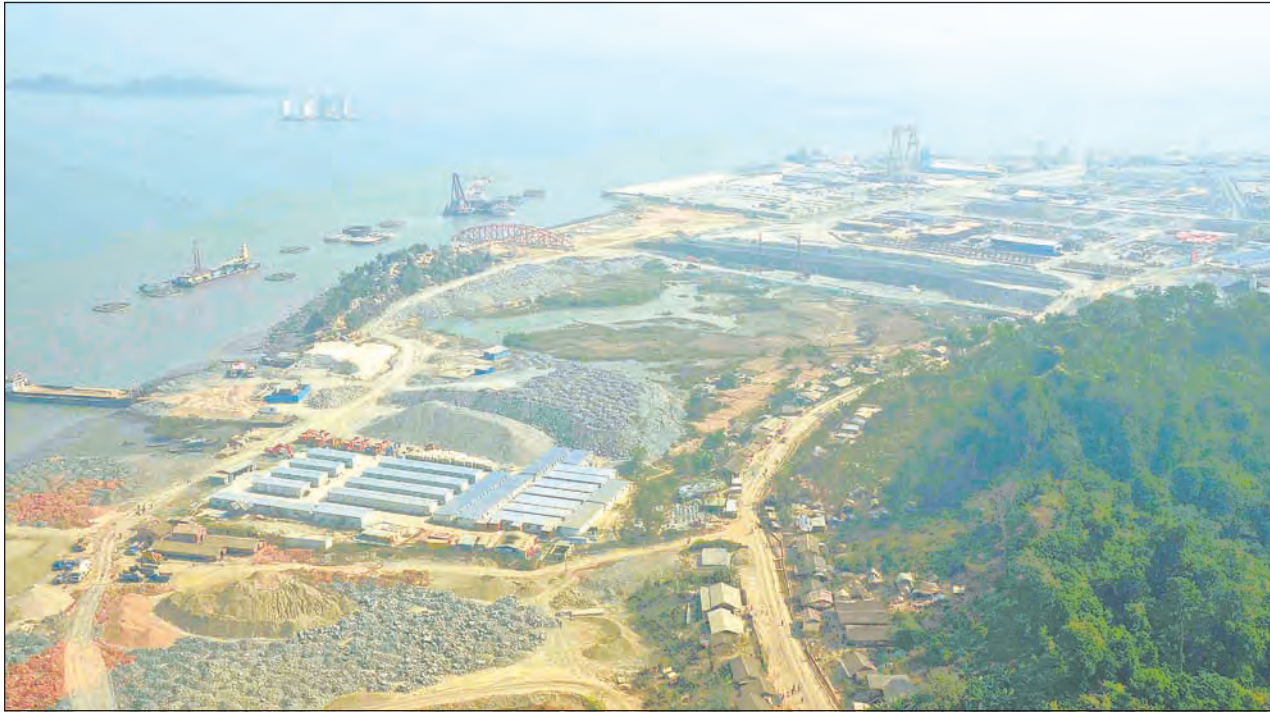
An aerial view of Myanmar-China oil and natural gas pipeline project in Ma-de Island in Rakhine State. (News on page 1)—MNA
