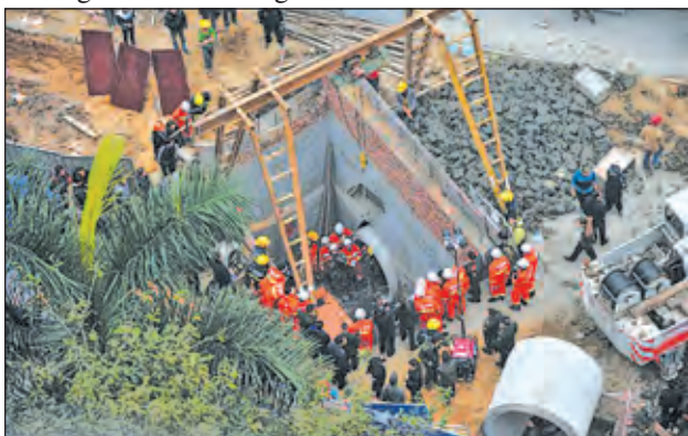
Rescuers work at the scene of a cave-in accident in Nanning, capital of south China's Guangxi Zhuang Autonomous Region, on 2 Jan, 2013. The tunnel of a metro line under construction in Nanning collapsed Wednesday afternoon, trapping three workers. Two have been rescued and one still trapped. —XINHUA
