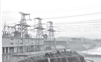
Photo taken on 13 July, 2012 shows the power transmission lines of the Three Gorges Dam in Yichang, central China's Hubei Province. As the second flood peak of this year passed, the Three Gorges power station started to operate at full capacity after its 32 turbine generators were all put into use on Friday. XINHUA
