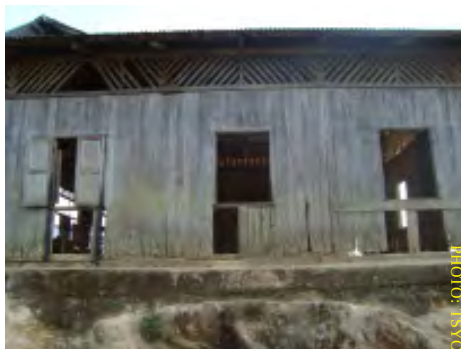
School in urgent need to repair
