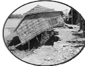
Bank erosion and damage to housings
