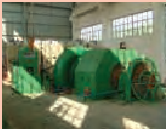
Mali hydroelectric plant
