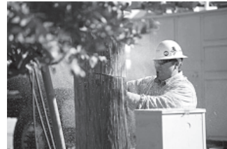
A utility worker saws down a damaged power line on Live Oak Ave, two days after severe wind storms caused major damage in Temple City, Calif, on 3 Dec, 2011.
