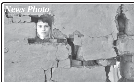
A boy looks through a damaged wall of his house after brief quakes affected the village of Tiguilotal in the municipality of El Carmen, some 163km (101 miles) east of the capital of San Salvador 26 November, 2011. More than 700 slight to moderate earthquakes hit an area in eastern El Salvador in a 24-hour period, damaging dozens of homes but hurting no one.—XINHUA
