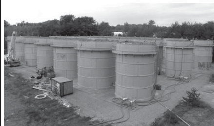
In this 27 May, 2011 photo released on 2 June, 2011 by Tokyo Electric Power Co (TEPCO), temporary storage tanks for low-level radioactive polluted waters used for temporary cooling system in Fukushima Daiichi nuclear power plant in Okuma, Fukushima prefecture, northeastern Japan, are shown. The nuclear facility was crippled when a huge tsunami generated by a magnitude 9.0 earthquake hit Japan on 11 March.—INTERNET
