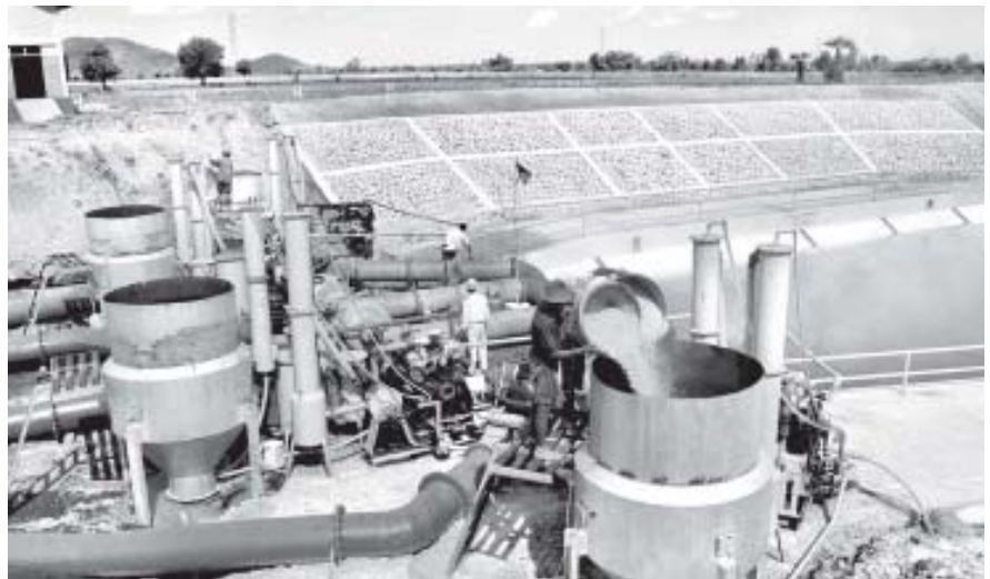
Paddy husk-fired gasifiers.
