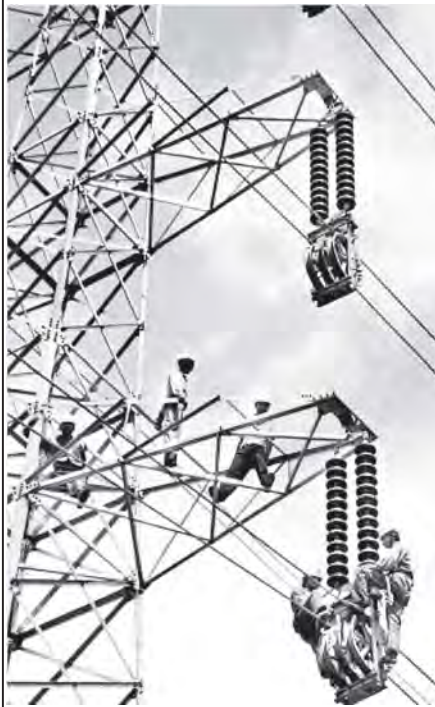
Power grids being lined up.
