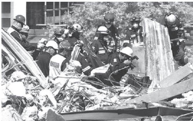
Emergency services work to remove a body from the site of the CTV building in Christchurch, New Zealand, on 24 Feb, 2011, after the city was hit by a 6.3 magnitude earthquake Tuesday.—INTERNET
