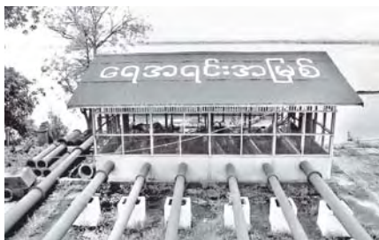
Letpanchepaw River Water Pumping Station.
