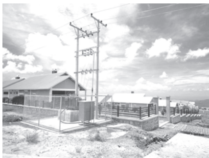
Transformer is ready to supply electricity.
