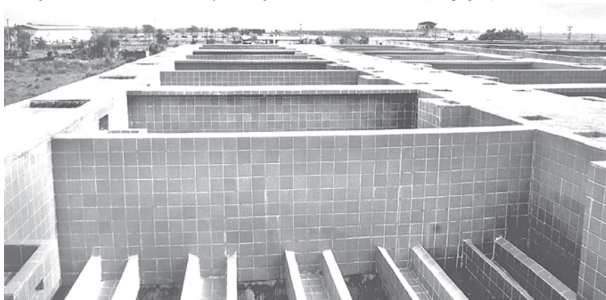
Water tanks of Ahtayu Water Supply Station of Yangon Water Supply Project (Ngamoeyeik) second phase.
