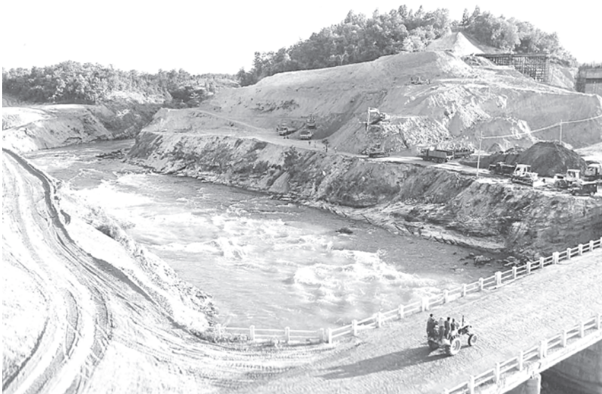
Mone Creek is blocked temporarily and the diversion drain is supplying water to farmlands.
