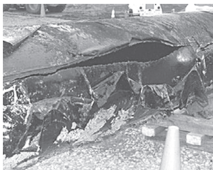
In this photo provided by the NTSB, a section of the pipeline that ruptured and spewed oil into a southern Michigan river is shown. The rupture extends approximately 6 1/2 feet longitudinally with the widest portion of the opening measuring 4 1/2 inches.
