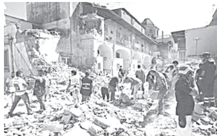
Italian firefighters and rescuers work at the site of an apartment building collapse in Afragola, near Naples, southern Italy, on
