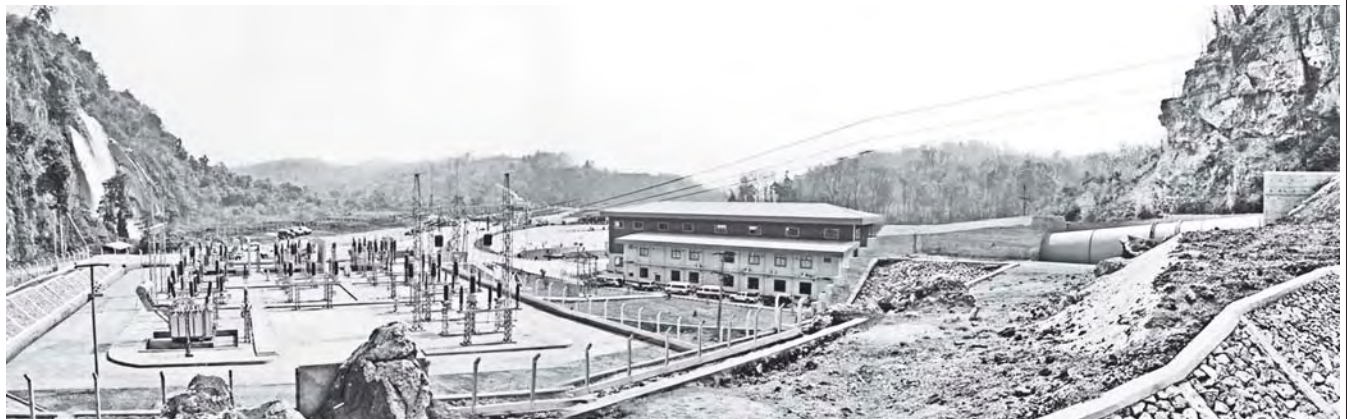
Switch Yards of Kengtawng Hydropower Plant.
