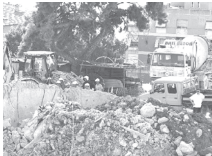
The metro construction site is seen after an explosion in Izmir, western Turkey, on 16 July, 2010. Two people were killed and four others injured on Friday when an air tank exploded at the metro construction site in Izmir.
